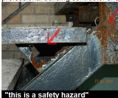
"this is a safety hazard"
