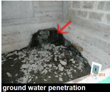
ground water penetration
